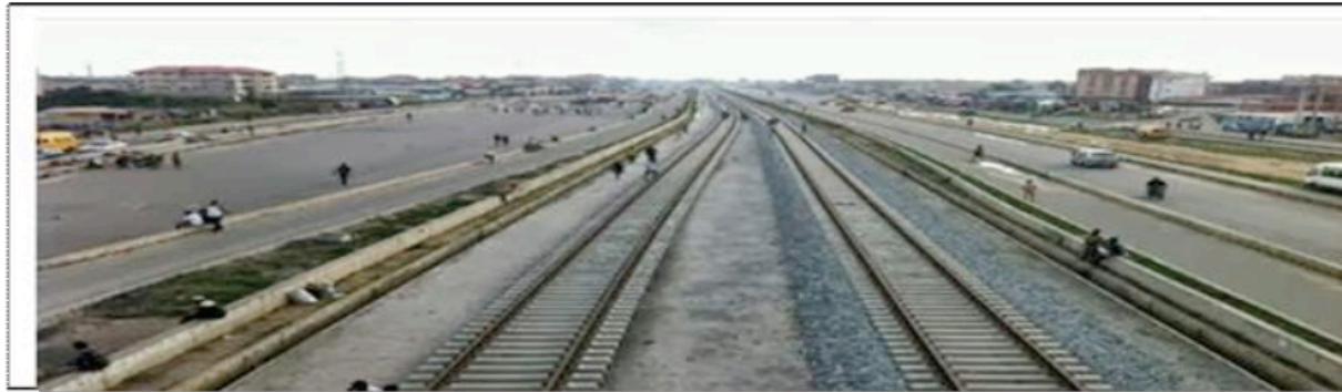
Figure 1: a: Prototype of Lagos–Badagry 10 Lane Expressways. b: Lagos–Badagry 10 Lane Expressways with wooden/concrete sleepers (Work in progress) below.
